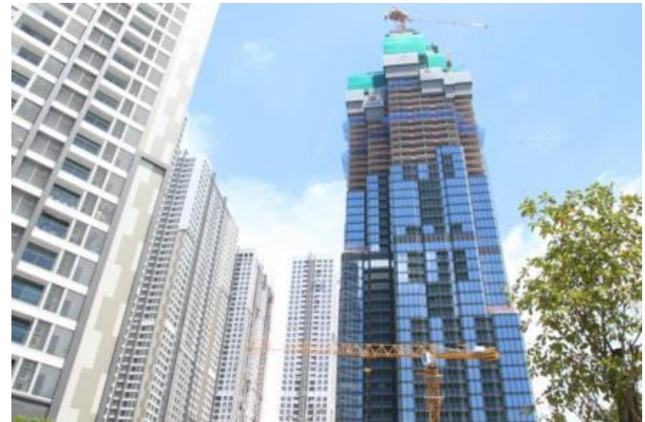
QH PLUS supplied structural steel for Landmark 81, the tallest tower in Vietnam.
